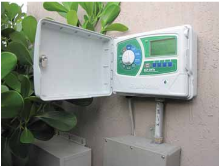
Figure 2. An example of an evapotranspiration control panel. Credits: Michael Gutierrez, UF/IFAS
