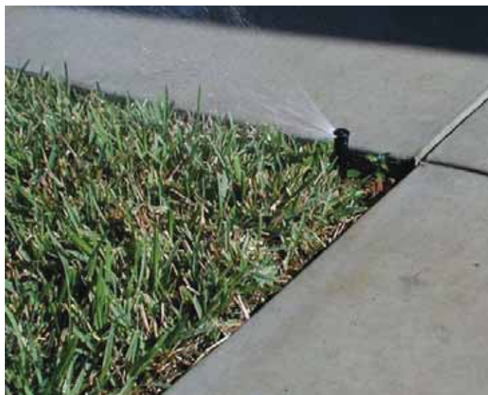
Figure 3. Fixed spray irrigation head.
